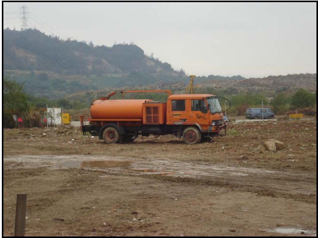
Figure 1 Water Truck stationed at Permanent Aviation Fuel Facility (PAFF) Construction Site (Photo: Leighton Contractors (Asia) Limited, November 2005)
