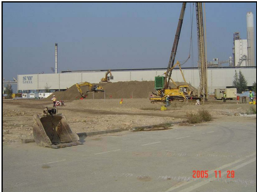
Figure 4 Sand surcharge at PAFF Construction Site (Photo: Leighton Contractors (Asia) Limited, November 2005)
