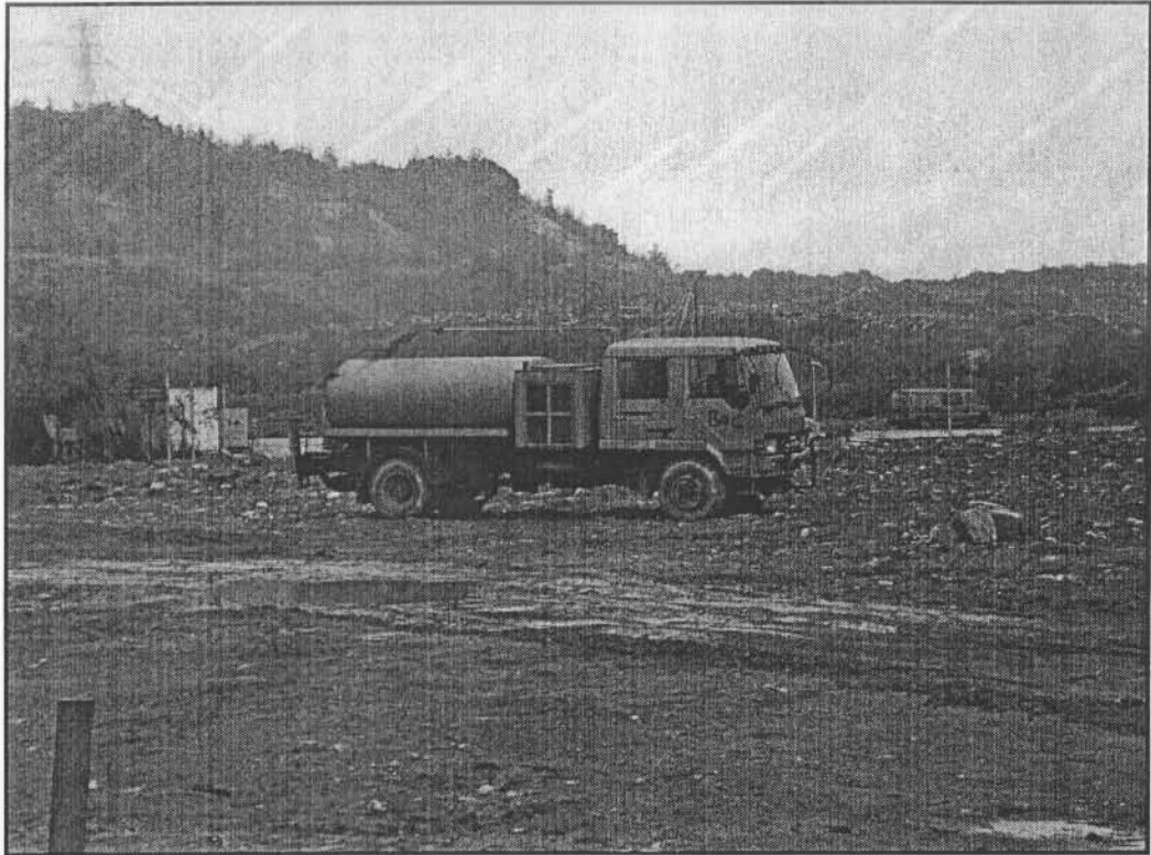
Figure 1 Water Truck stationed at Permanent Aviation Fuel Facility (PAFF) Construction Site (Photo: Leighton Contractors (Asia) Limited, November 2005)
